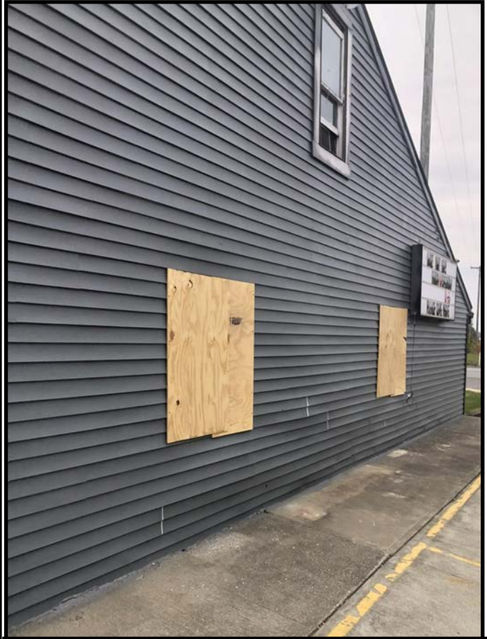
In October, the windows are boarded up in anticipation of the front door installation.
