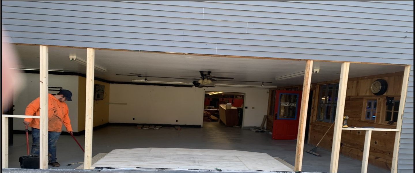
StoneBridge Operator and retired Contractor Bill Mattingly spearheaded the entire renovation. He was the lead carpenter on the entire renovation.
